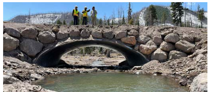
Figure 3: Completed bottomless arch culvert with locally sourced stone applied to headwalls and stream grade control. Construction efforts are later supplemented with the planting flood resilient vegetation, such as willows, to reduce erosion, increase bank stability and restore habitat for fish and wildlife. Credit: Dave Turk, AECOM
