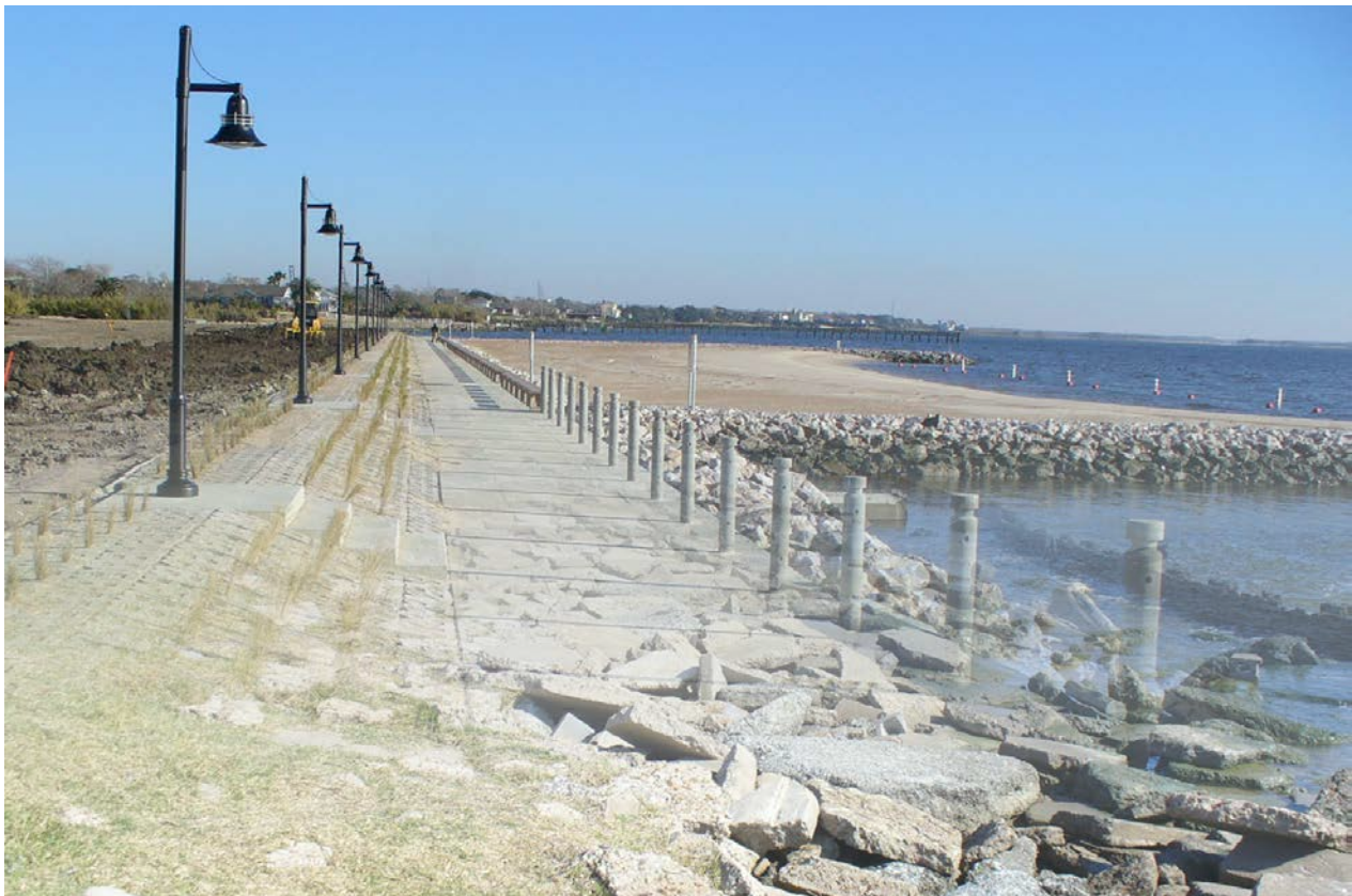
The Sylvan Beach project in La Porte, TX is a hybrid solution that created a community beach park using sand as a nature-based feature held in place by engineered rock groins.
